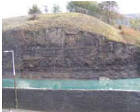
Rocks in Godley Cutting which have been cleared of vegetation and will remain exposed.
